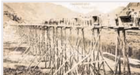
Embankment filling work behind the Bad Hofgastein railway station. The scaffolding in left in the embankment after the placement operation
