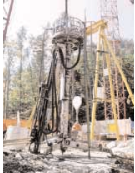
Headframe and drill rig
