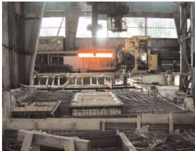
With the plant working normally space is in short supply
