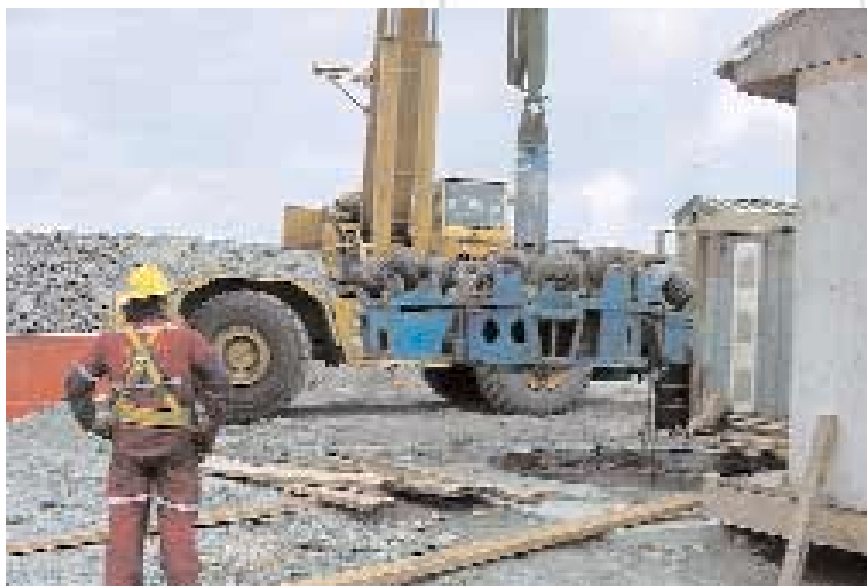
Dismantling the Sandvik reamer head (diameter 3.0 m) after completion of the raise
