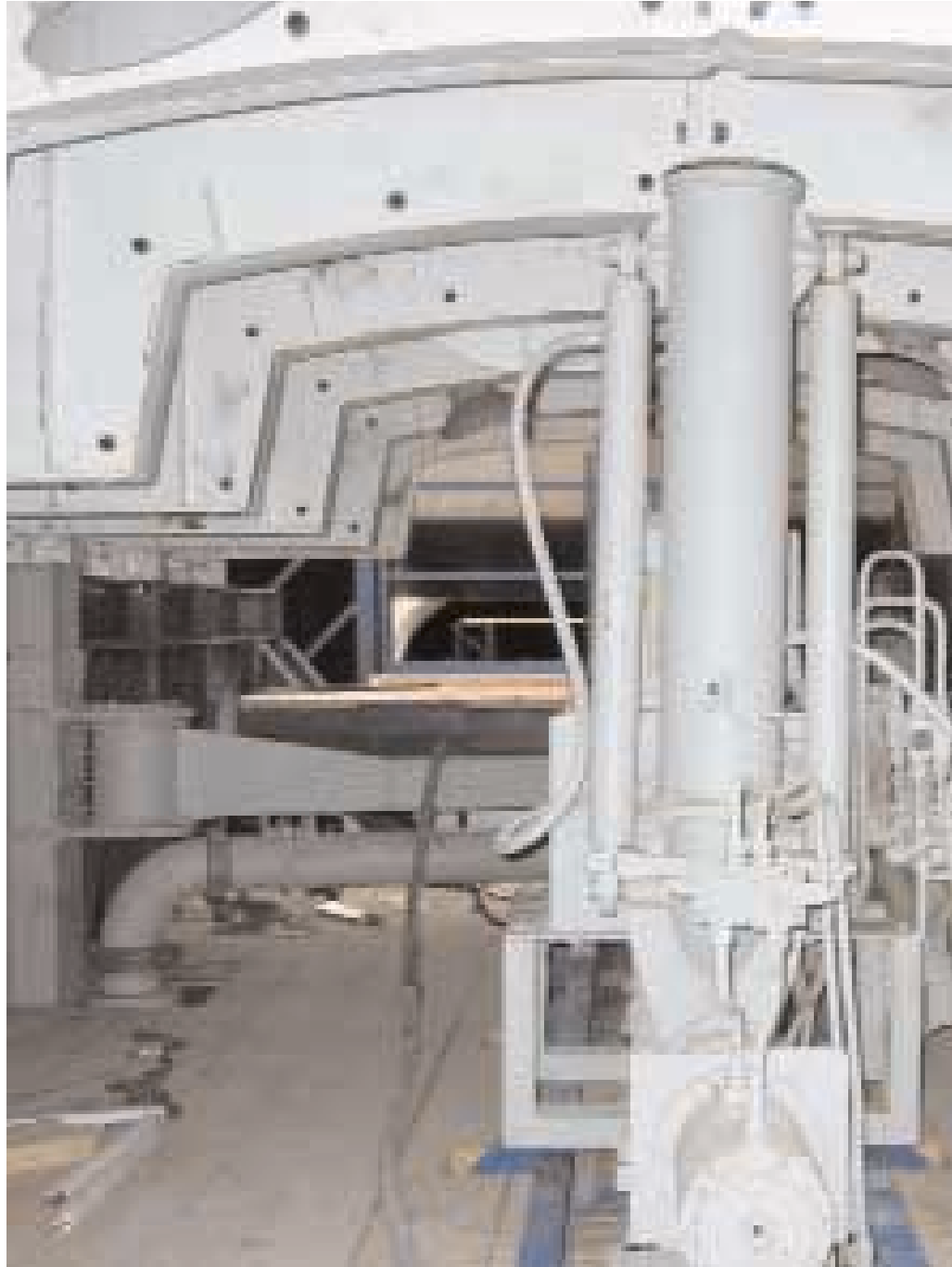
Tunnel crown viewed from below with sliding support brackets and hydraulic tunnel concreting machine
