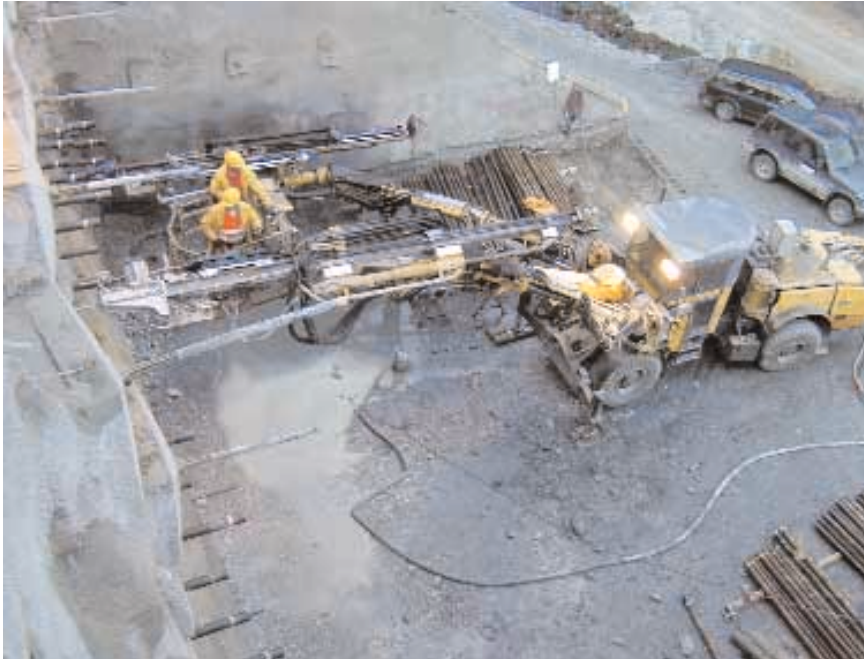
Erecting the first screenpipe at the west portal of the Birgl tunnel
