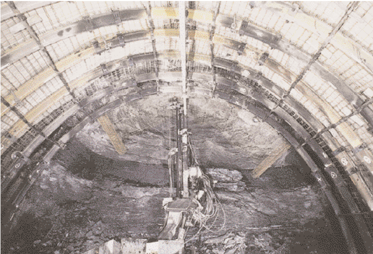
Bolting in the roof with compact jumbo drill. The two in-seam dirt-bands are clearly visible (reference roadway)
