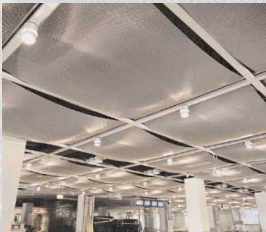
30.000m 2 of metal-fabric ceiling as part of the overall fire protection system
