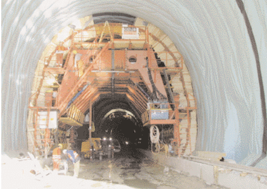
Shuttering times are reduced by use of arch forms, which allow bolt-free working
