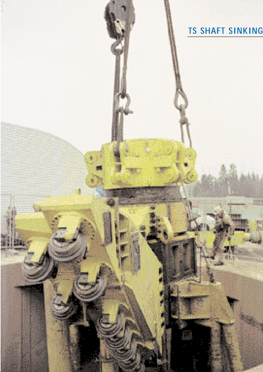
Assembly of the Wirth SB VII shaftboring machine, mounting of the part-assembled boring head
