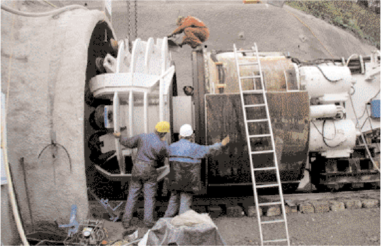
Fitting the drill head to the tunnel boring machine at the gallery mouth
