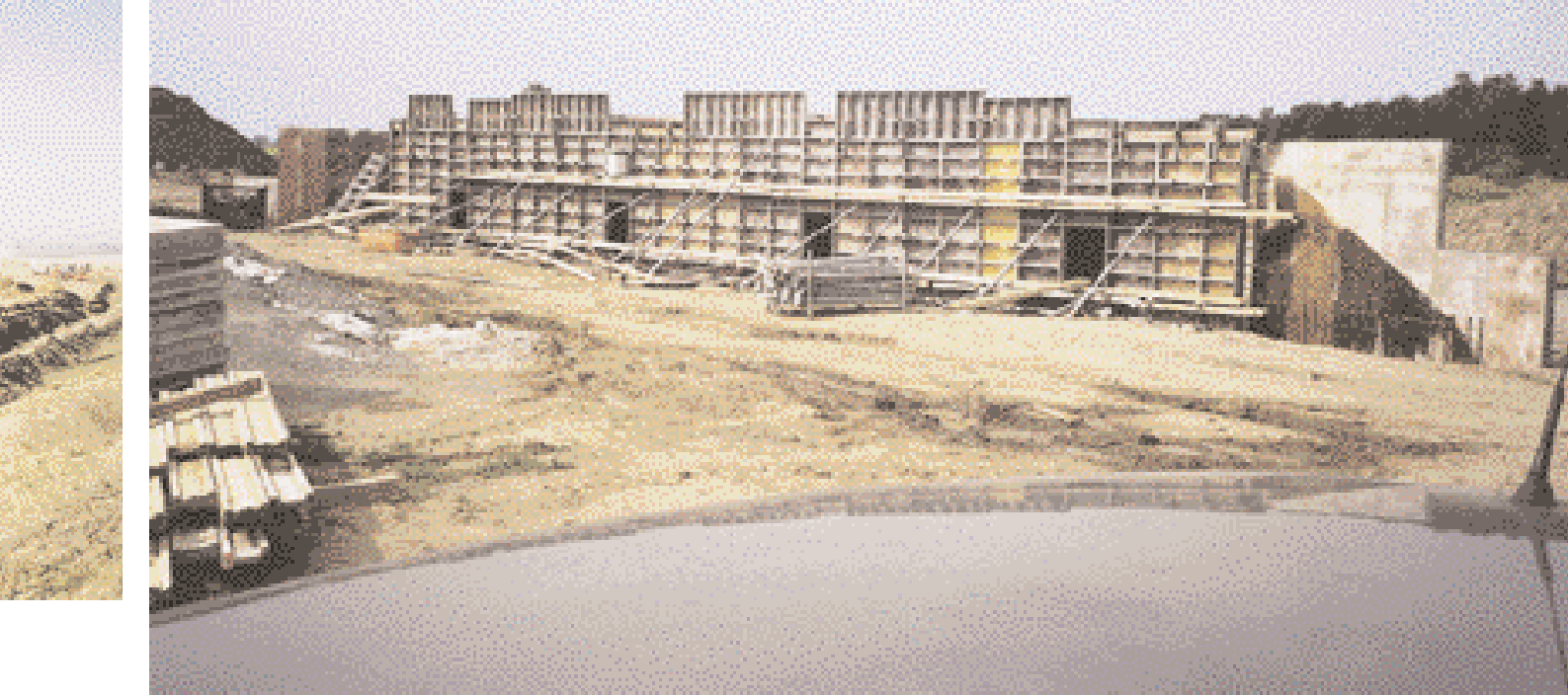
Front formwork (average height 4 metres) and 32.5 metre-long drainage culvert no. 4 (diam. 1800 mm), which crosses the national highway at an angle of 32°
