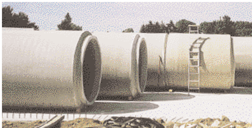
Assembly of steel-concrete pipes for drainage culvert no. 4 (weight of each pipe: 10 tons)
