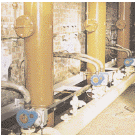
Gas collection system
