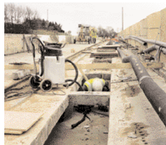
Photograph showing parapet strengthening works on Pleasley Lane Overbridge on the M1 Motorway.
