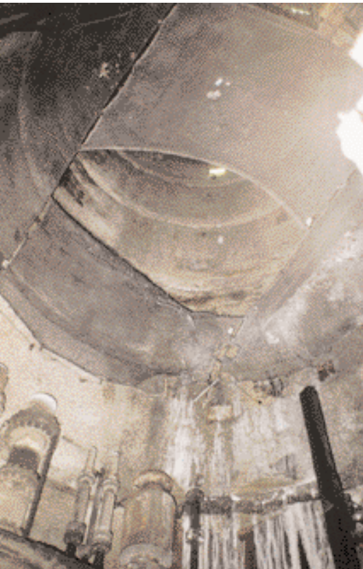
View of overhead protection system
