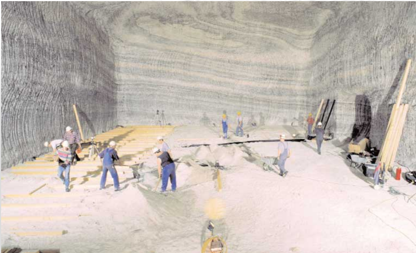
Concert hall after excavation, with workmen engaged in laying the wood flooring
