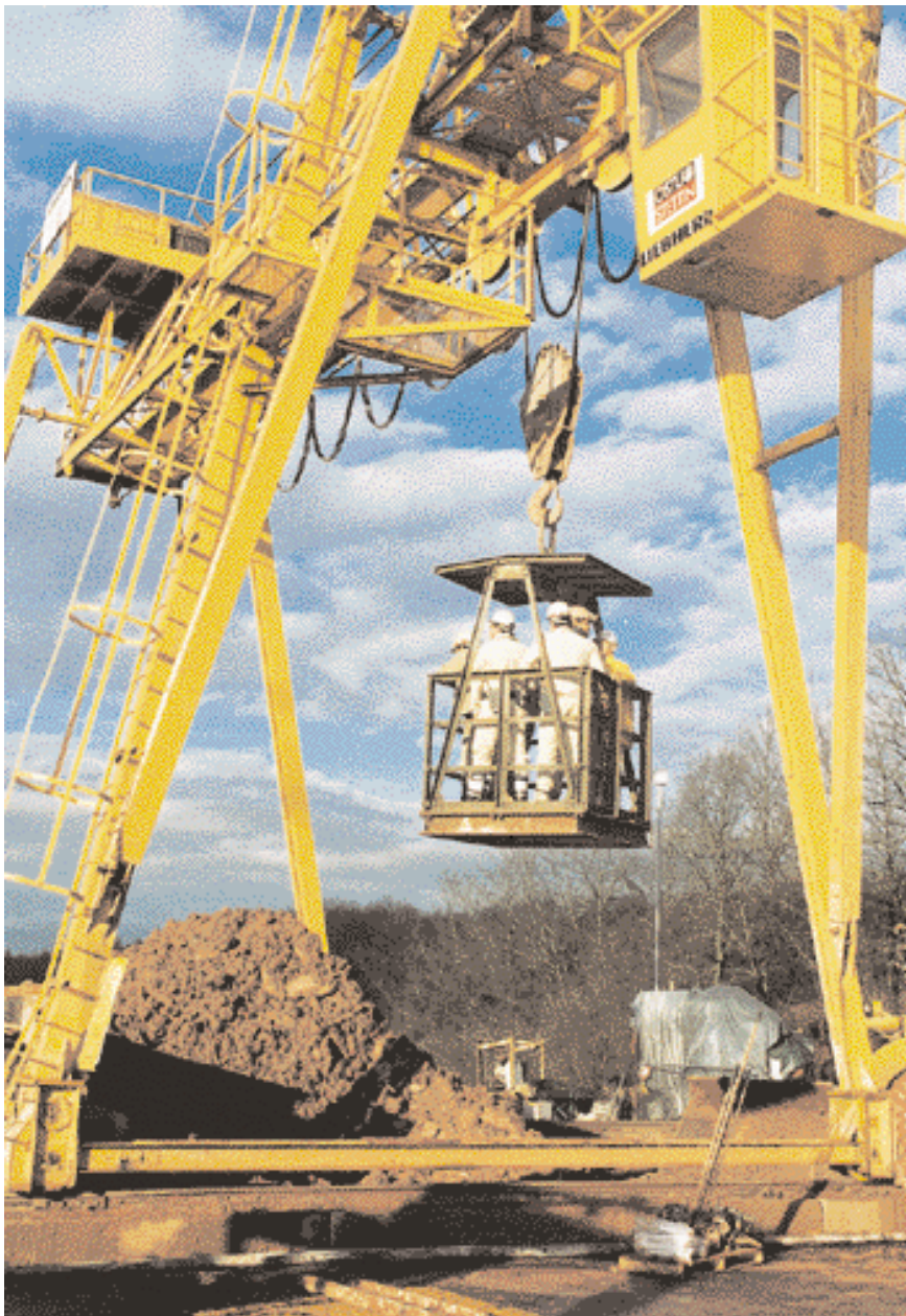
Manwinding cage transports personnel in foreshaft section
