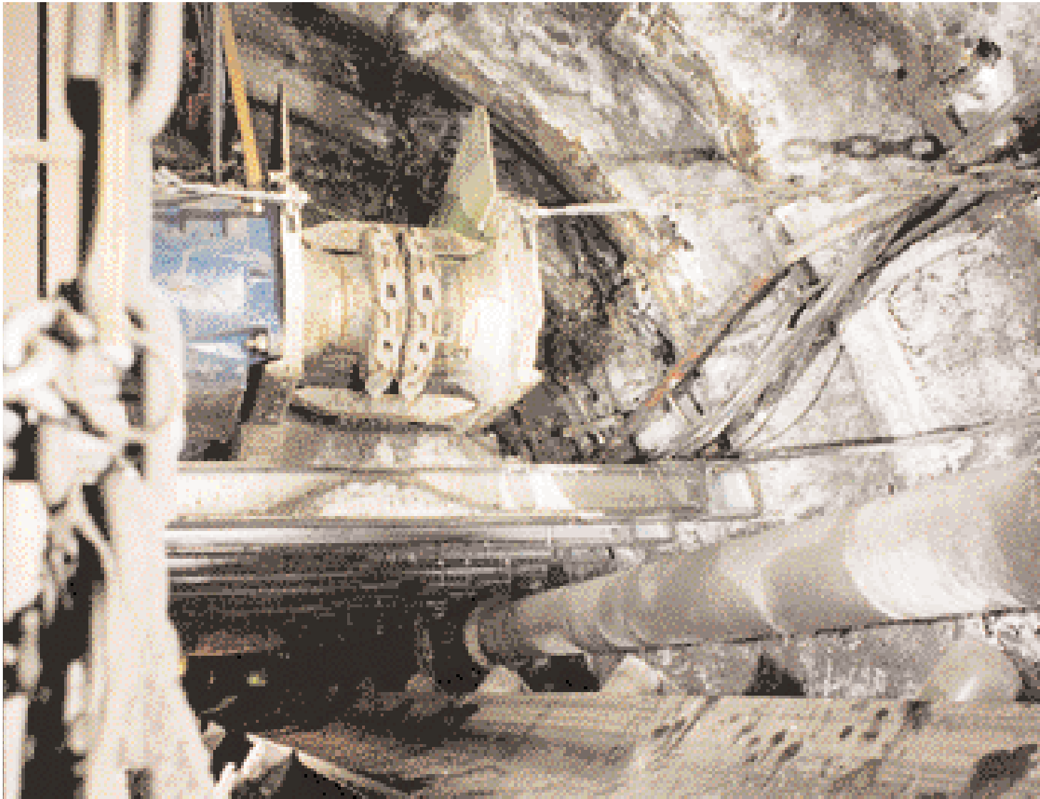
Excavated debris is delivered by chain conveyor to the main belt on mine level 5
