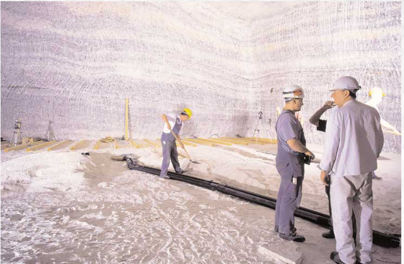
Concert hall after excavation, with electricians engaged in installing the electrical installations
