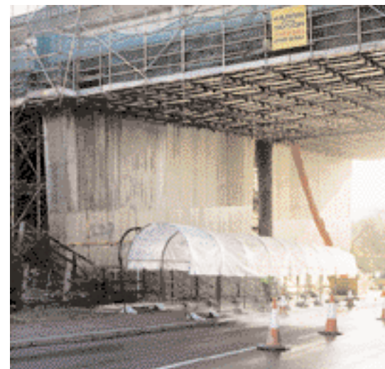
Photograph showing temporary scaffold to facilitate bridge strengthening works to Whitehill Lane Underbridge, M1 Motorway complete with temporary cover to pedestrian footpath.
