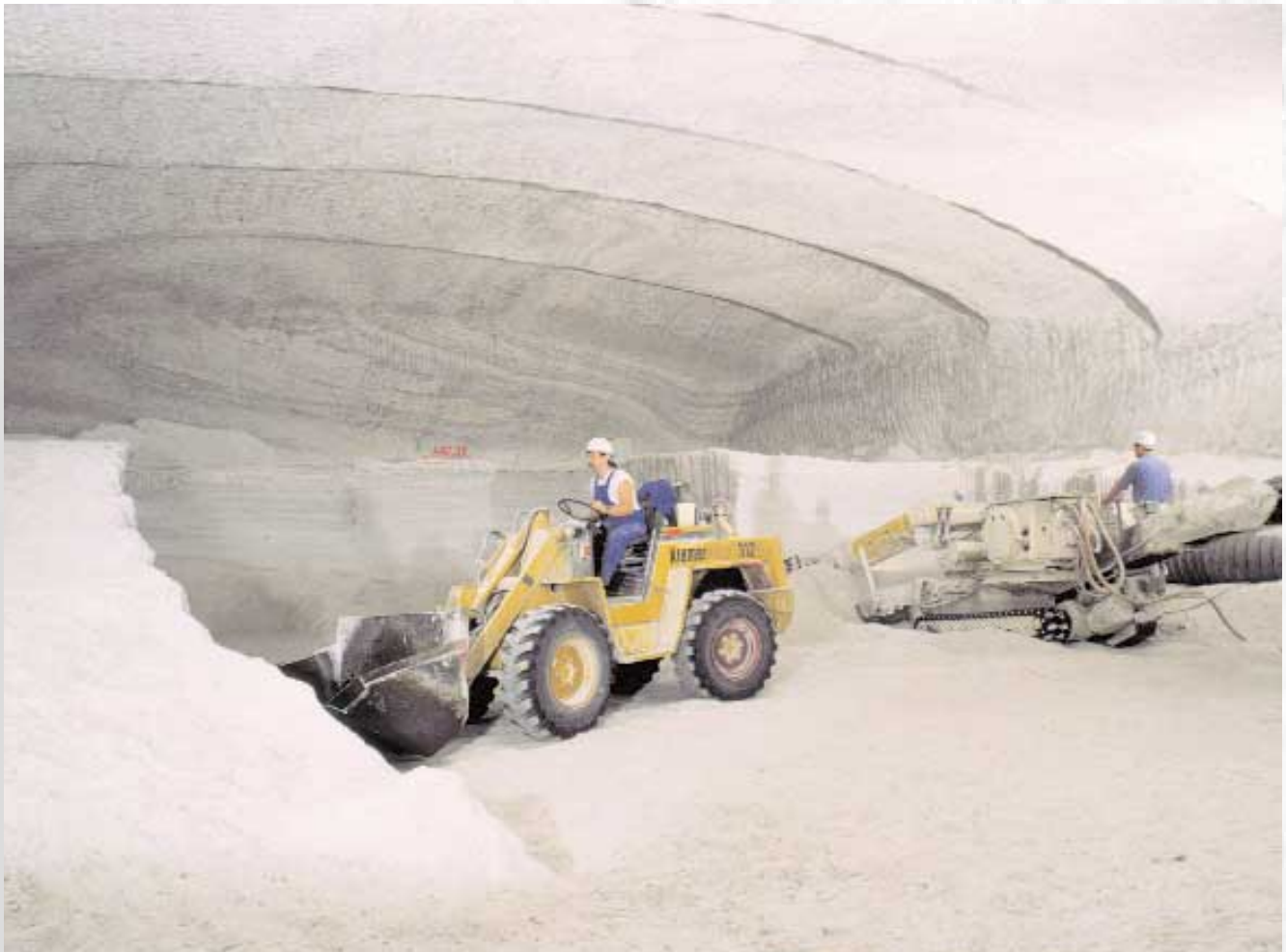
Excavation of the second and third slice (after completion of roof profile)
