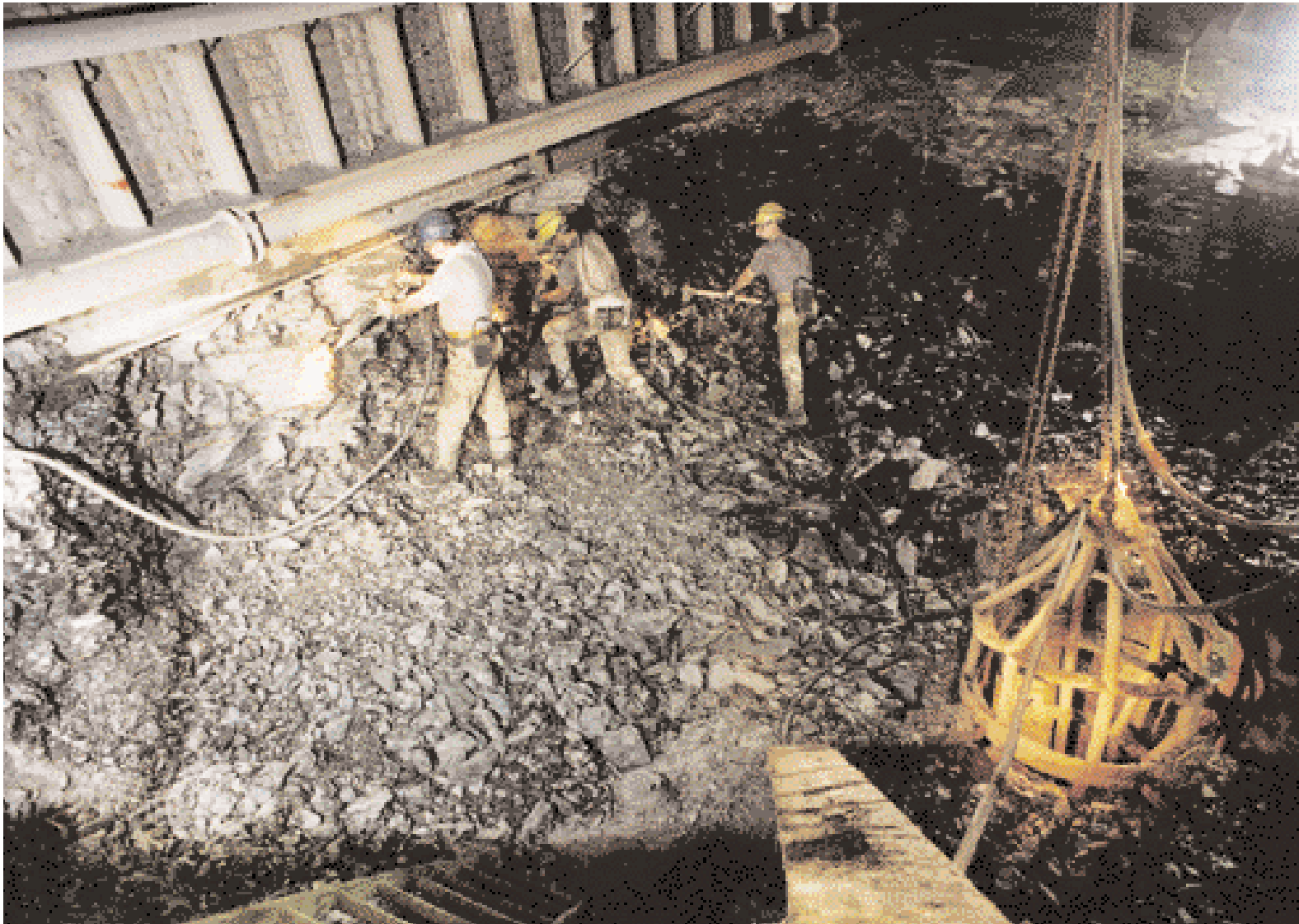
Shaft sinking below the roadway: collar excavation extends well below the arch supports
