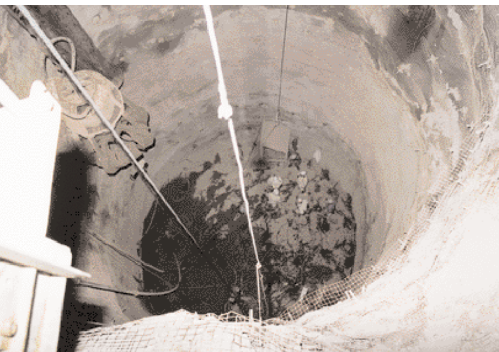
Shaft sump is excavated from the solid by drilling and firing and then supported by rockbolts and wire mesh
