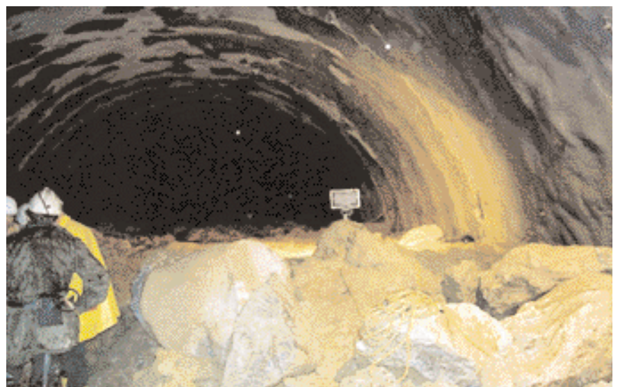
Material washed out into the tunnel
