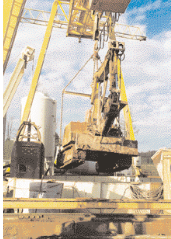
10-tonne excavator for foreshaft section can be raised and lowered at will
