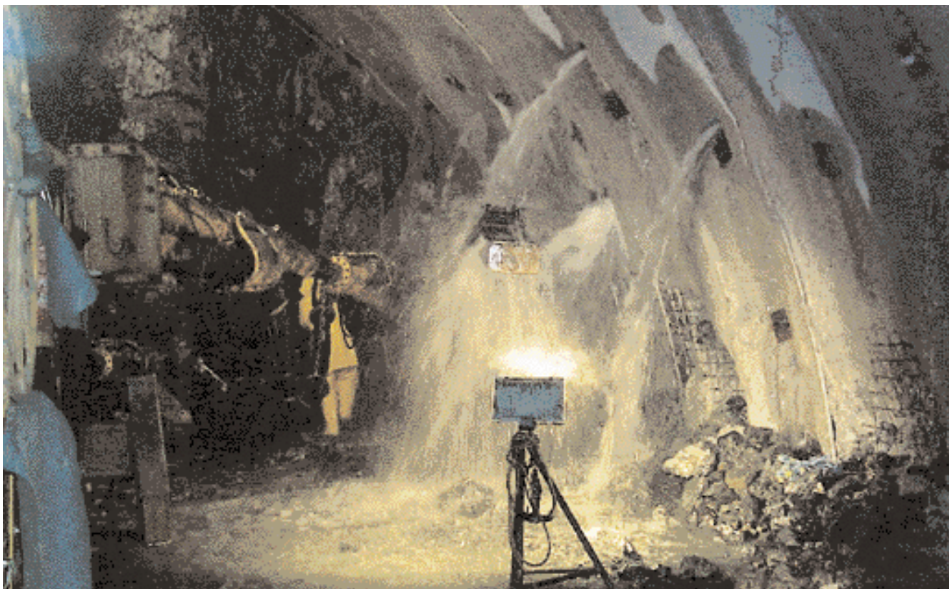
Water inflow in the crown drivage zone
