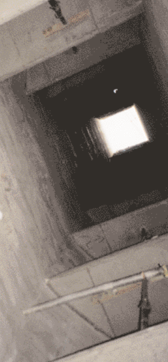
Emergency exit shaft NA4 after installation of landings, viewed from shaft bottom; the pre-fabricated stairway sections are lowered in through the surface opening in order to allow the landings to be connected together
