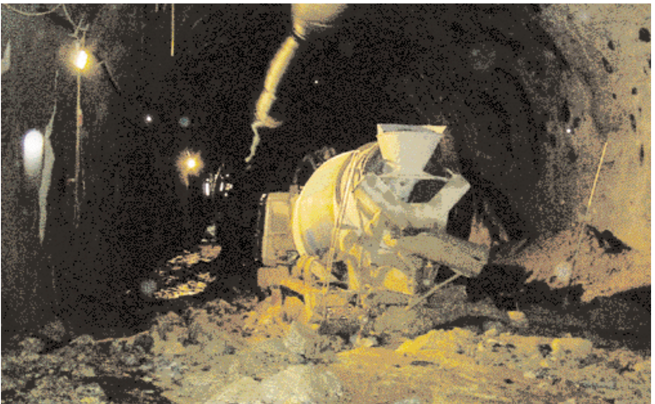
Mobile concrete mixer entrained by the flow of mud and rock
