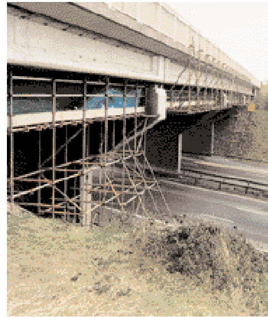
Photograph showing temporary scaffold to facilitate bridge strengthening and parapet works to Pleasley Lane Overbridge over the M1 Motorway.
