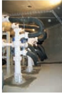
Brine heads in the freeze cellar at number 1 shaft
