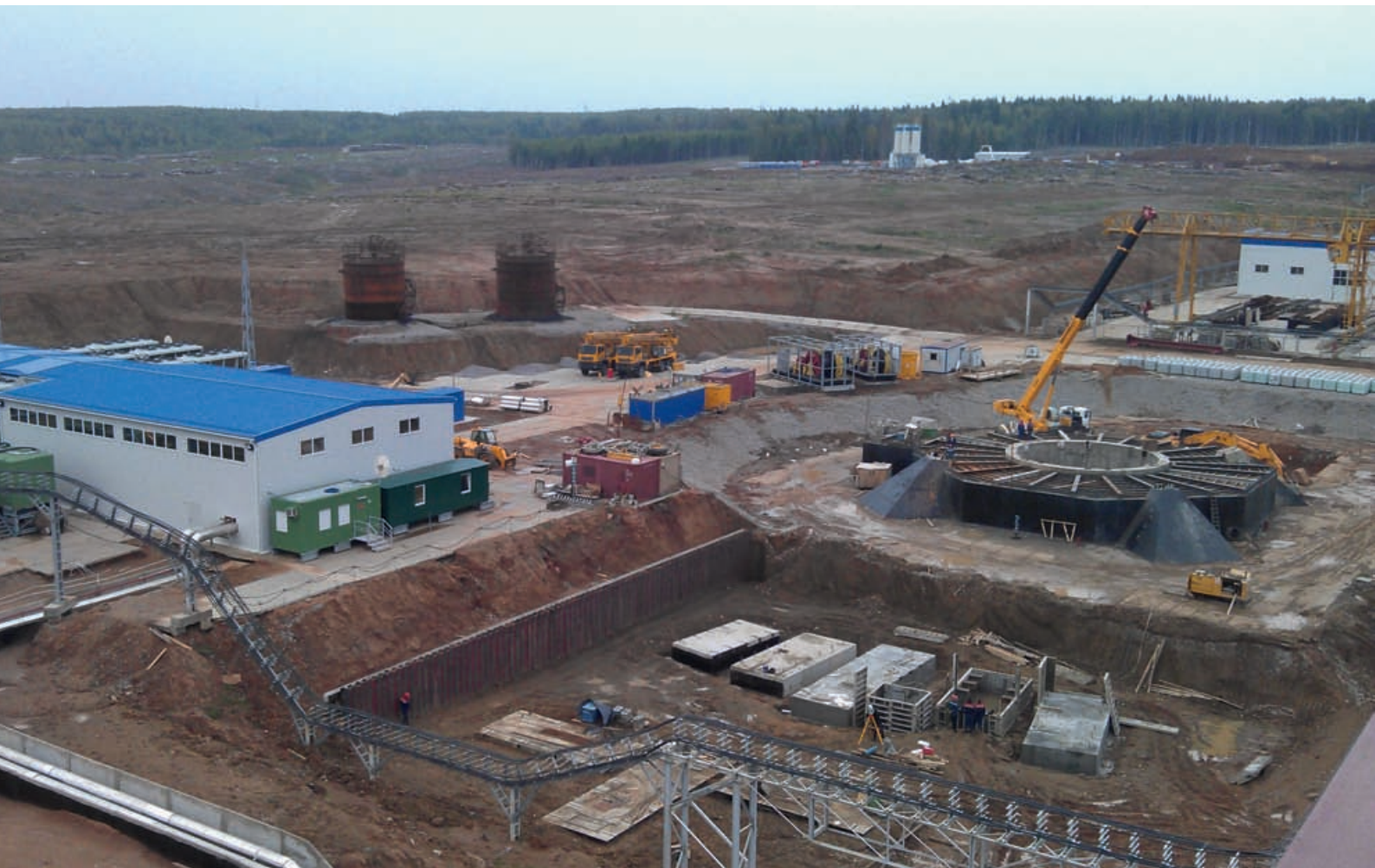
View of the freeze plant and state of progress at number 2 shaft
