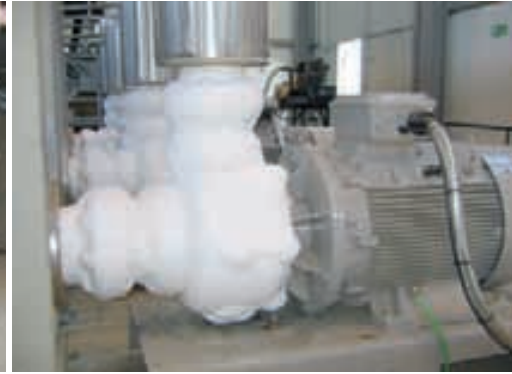
Ice build-up on the brine pumps
