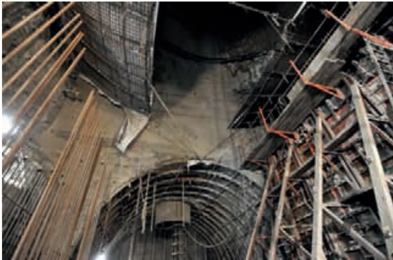
Constructing the walls for the hopper support surfaces, overhead screens to prevent contamination of the reinforcement
