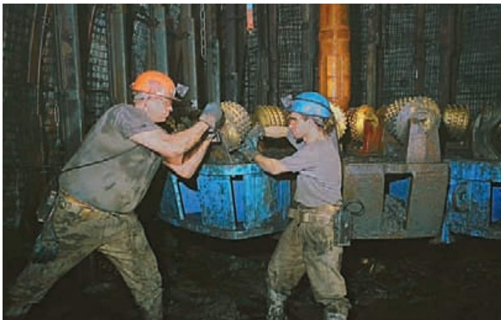
Assembling of the reaming head at the bottom of the blind shaft
